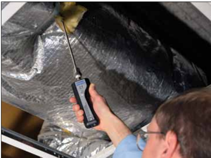
Figure 1: Measuring air duct temperature with UWBT-RTD-M12
