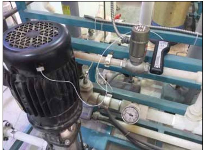
Figure 7: SA1-RTD sensor mounted to pump motor
