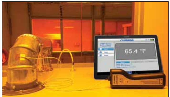
Figure 3: UWBT-RTD-TB monitoring exhaust gas temperature
