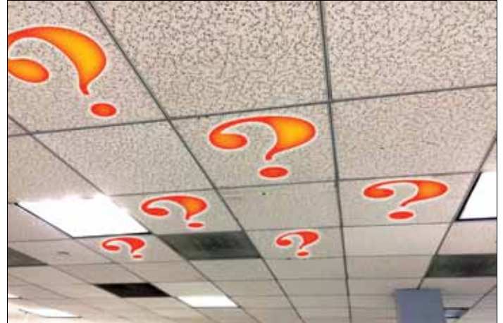
Figure 4: Which ceiling tile holds the UWBT transmitter?
